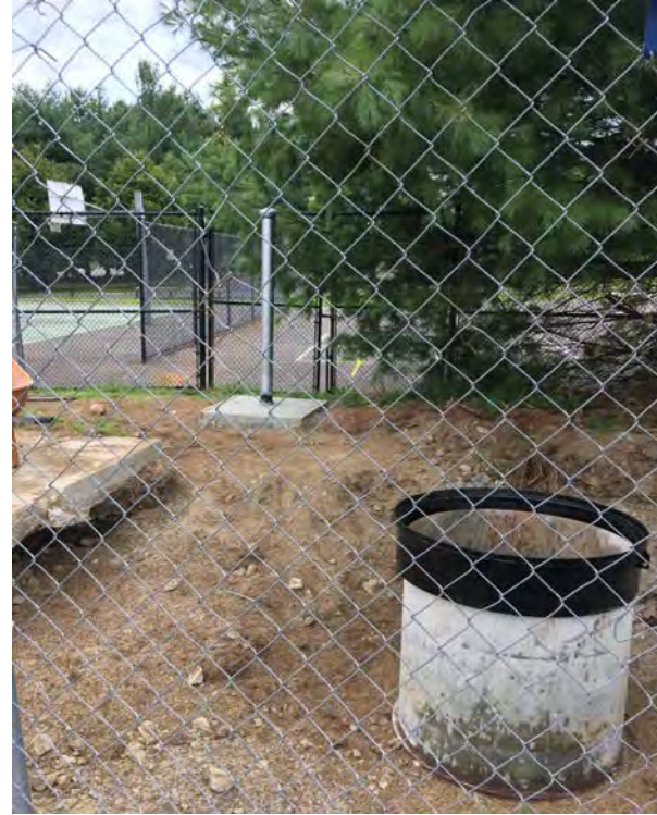
New tank Pressure vent
