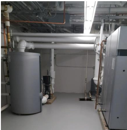
New gas fired burners at NMS
