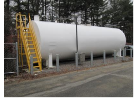
20,000 gallon oil tank located at NHS
