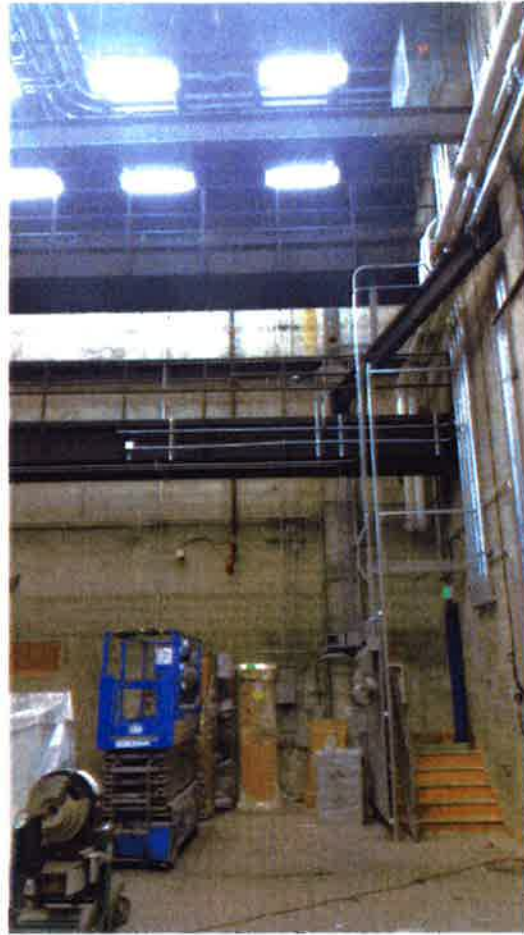
Rigging Galleries Catwalks (9/8/2017)
