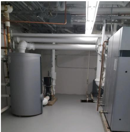
New gas fired burners at NMS
