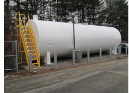
20,000 gallon oil tank located at NHS
