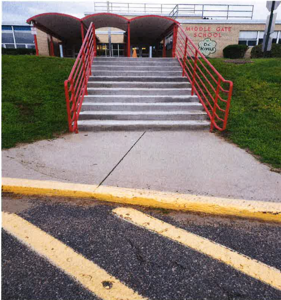
Middle Gate – Repair concrete steps in parking lot
