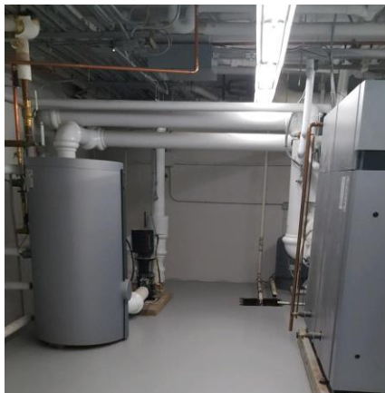
New gas fired burners at NMS
